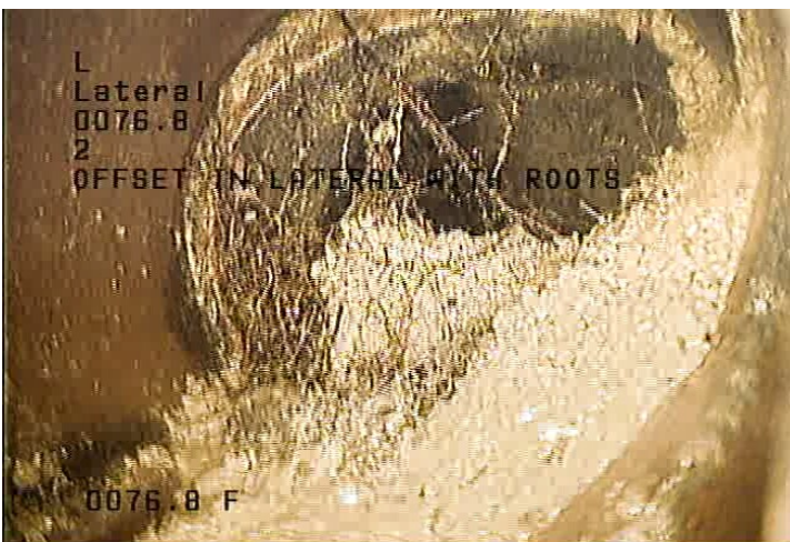
L - Lateral @ 76.8 ft. OFFSET IN LATERAL WITH ROOTS
