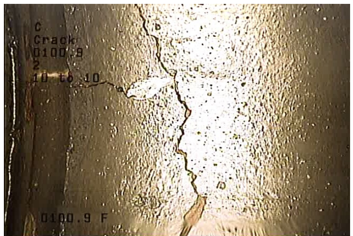
C - Crack @ 100.9 ft.
