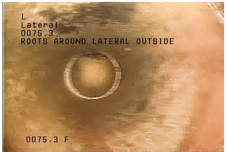
L - Lateral @ 75.3 ft. ROOTS AROUND LATERAL OUTSIDE
