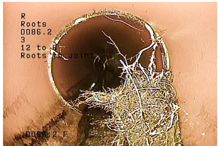
R - Roots @ 90.6 ft. Roots in joint
