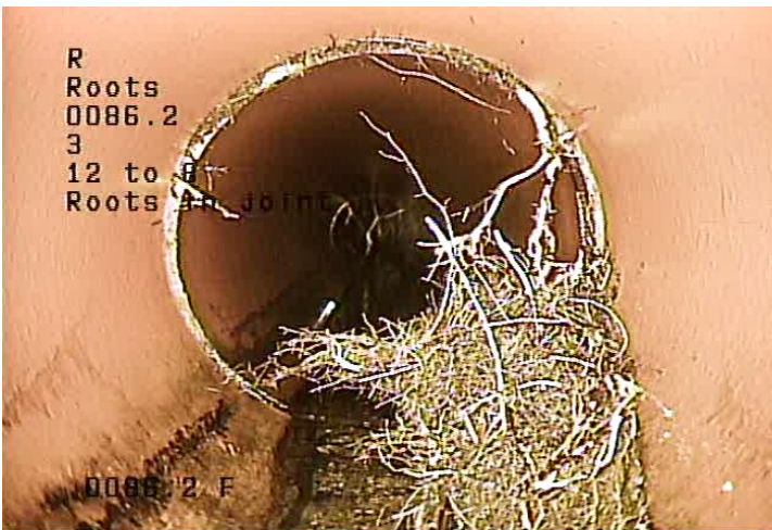
R - Roots @ 86.2 ft. Roots in joint
