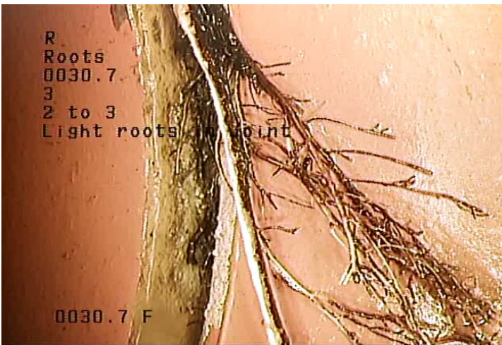
R - Roots @ 30.7 ft. Light roots in joint
