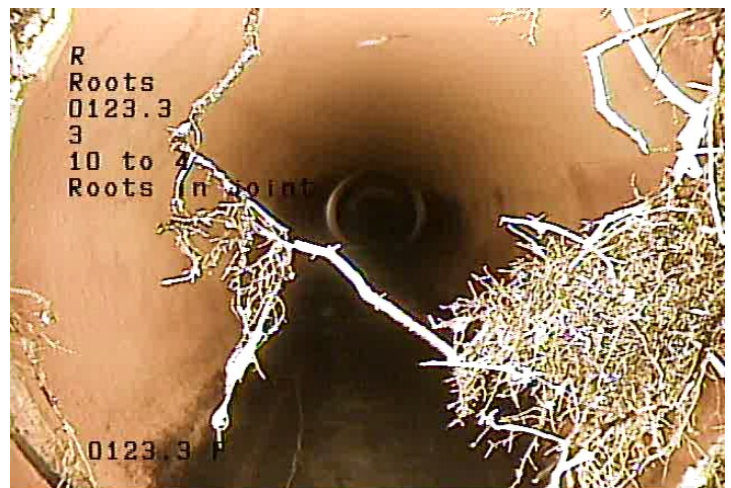
R - Roots @ 123.3 ft. Roots in joint
