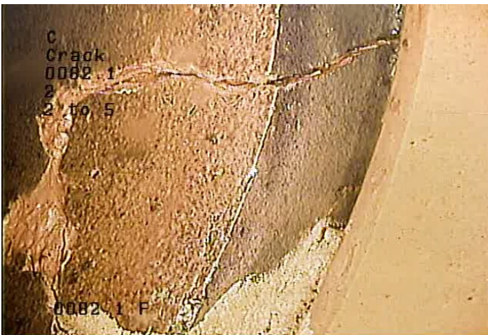
C - Crack @ 82.1 ft.
