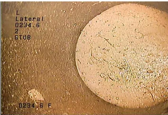
L - Lateral @ 234.6 ft. STUB
