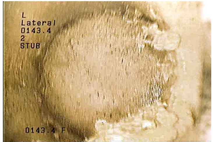
L - Lateral @ 143.4 ft. STUB
