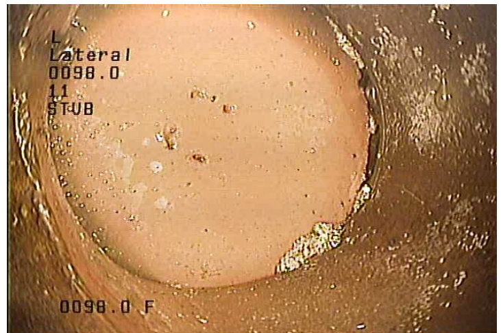
L - Lateral @ 98.0 ft. STUB
