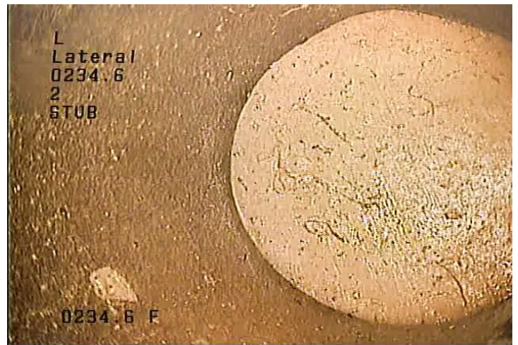
C - Crack @ 235.9 ft.
