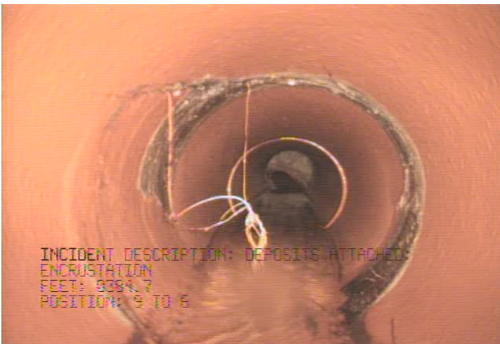
DAE - Deposits Attached: Encrustation @ 384.7 ft.
