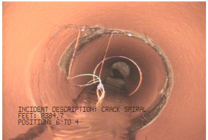
CS - Crack Spiral @ 384.7 ft.
