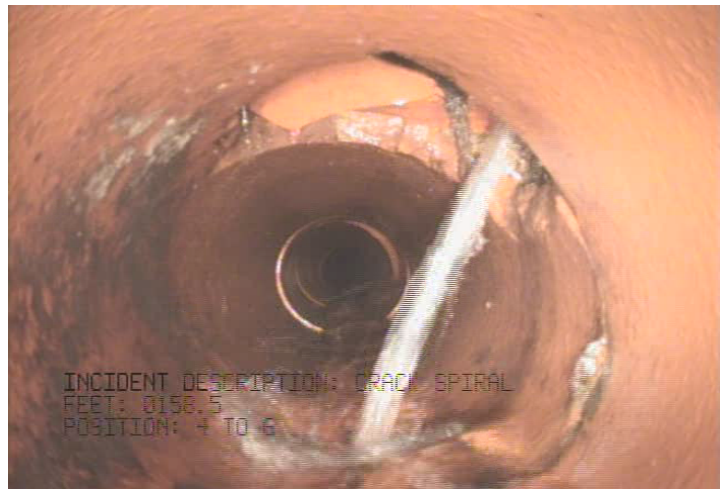
CS - Crack Spiral @ 158.5 ft.
