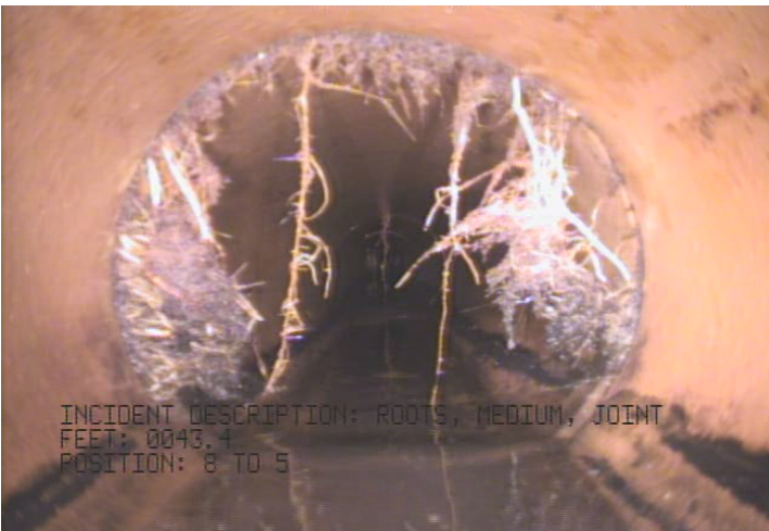
RMJ - Roots, Medium, Joint @ 43.4 ft.
