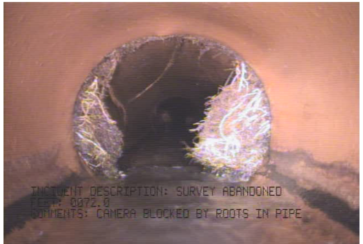
MSA - Survey Abandoned @ 72.0 ft. Camera Blocked By Roots In Pipe
