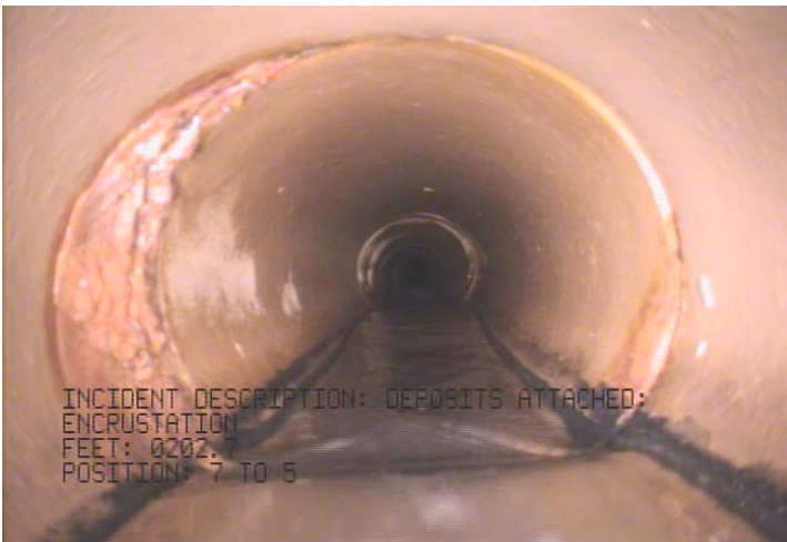
DAE - Deposits Attached: Encrustation @ 202.7 ft.
