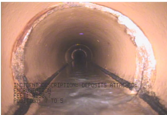
DAE - Deposits Attached: Encrustation @ 190.7 ft.
