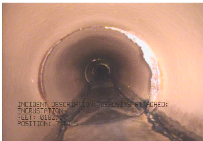
DAE - Deposits Attached: Encrustation @ 182.1 ft.
