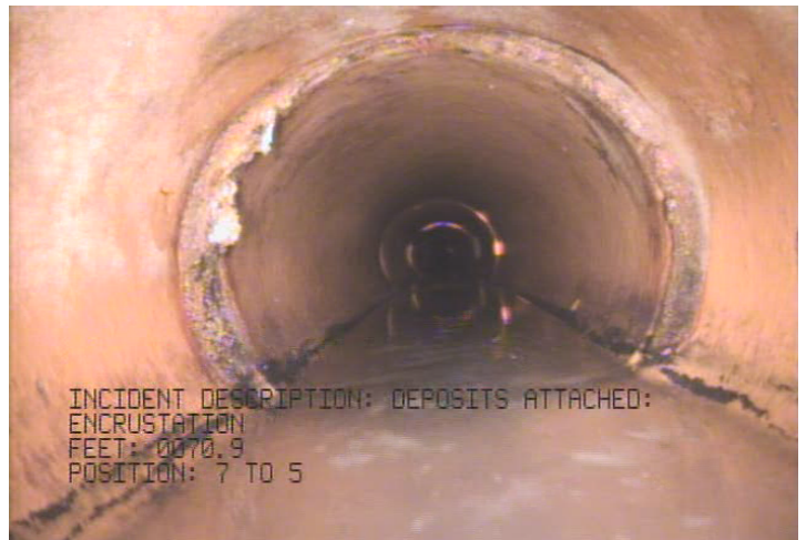
DAE - Deposits Attached: Encrustation @ 70.9 ft.
