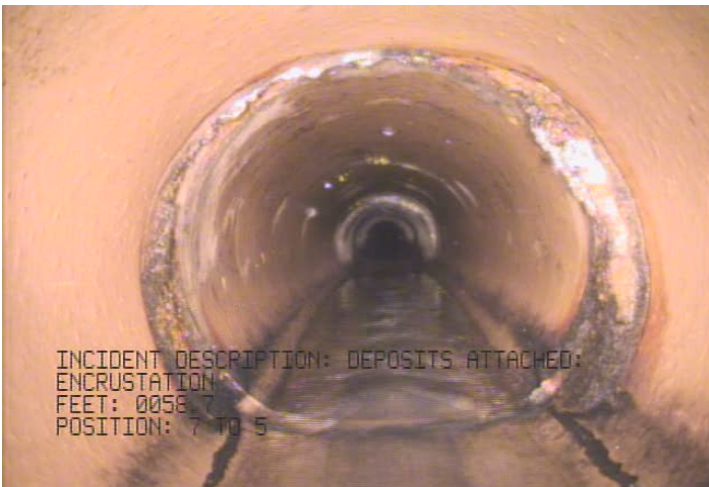
DAE - Deposits Attached: Encrustation @ 58.7 ft.
