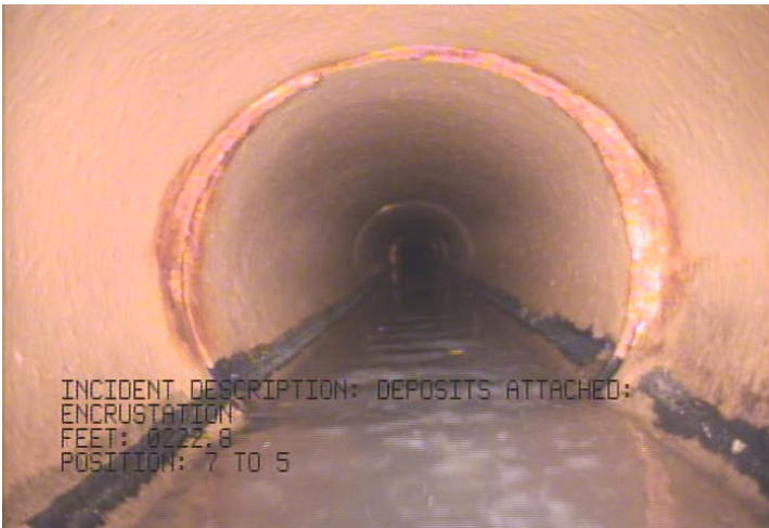
DAE - Deposits Attached: Encrustation @ 222.8 ft.
