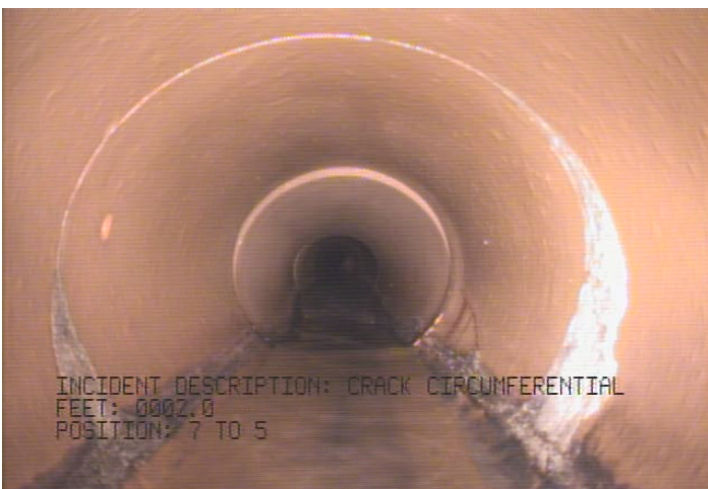
CC - Crack Circumferential @ 2.0 ft.
