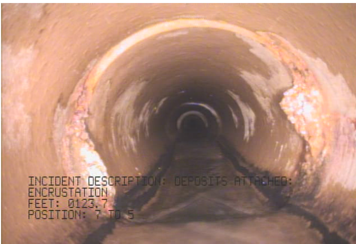
DAE - Deposits Attached: Encrustation @ 123.7 ft.
