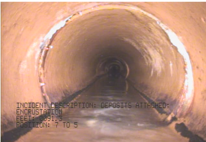
DAE - Deposits Attached: Encrustation @ 91.3 ft.
