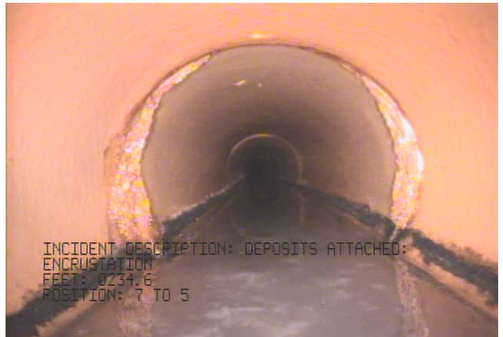
DAE - Deposits Attached: Encrustation @ 234.6 ft.
