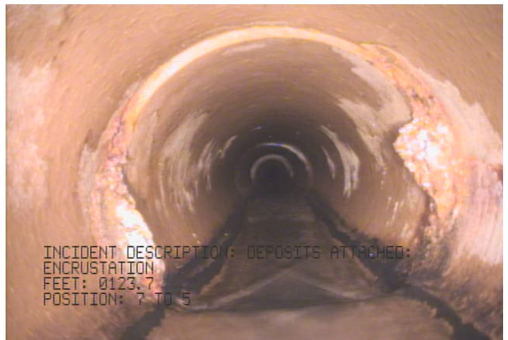
DAE - Deposits Attached: Encrustation @ 123.7 ft.
