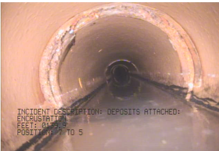
DAE - Deposits Attached: Encrustation @ 139.9 ft.
