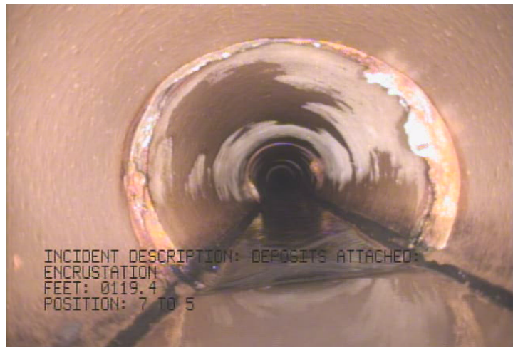
DAE - Deposits Attached: Encrustation @ 119.4 ft.
