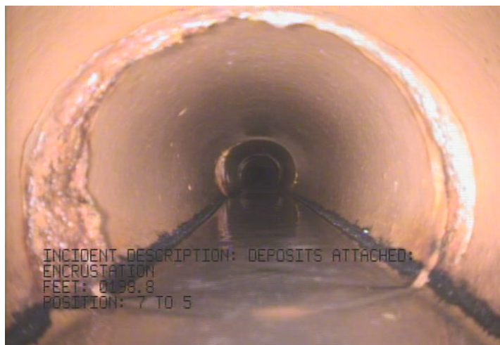
DAE - Deposits Attached: Encrustation @ 198.8 ft.
