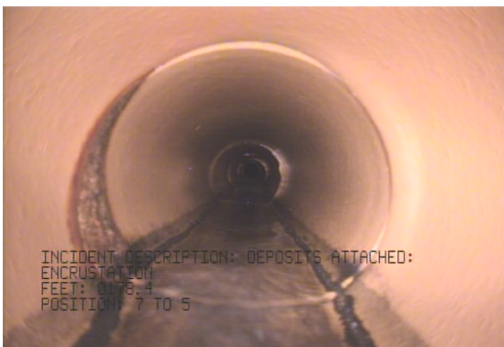
DAE - Deposits Attached: Encrustation @ 178.4 ft.
