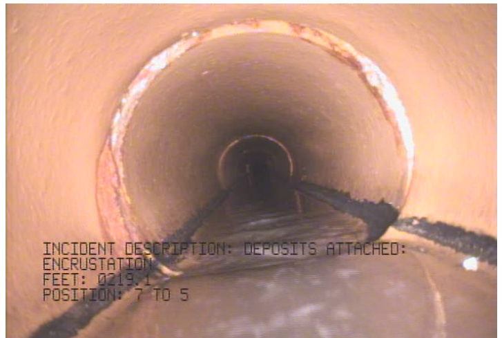
DAE - Deposits Attached: Encrustation @ 219.1 ft.
