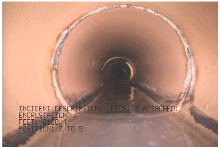
DAE - Deposits Attached: Encrustation @ 168.4 ft.
