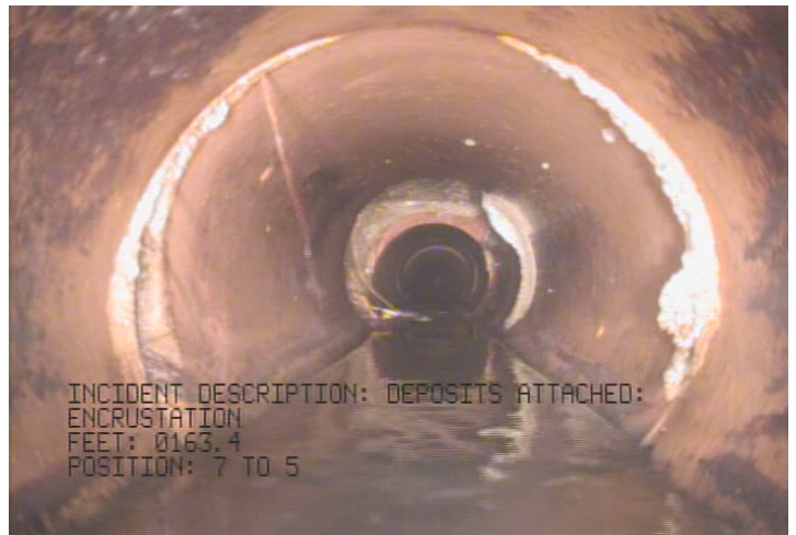
DAE - Deposits Attached: Encrustation @ 163.4 ft.
