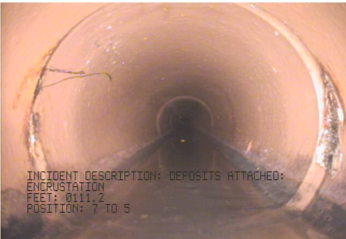
DAE - Deposits Attached: Encrustation @ 111.2 ft.
