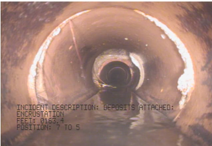
DAE - Deposits Attached: Encrustation @ 163.4 ft.
