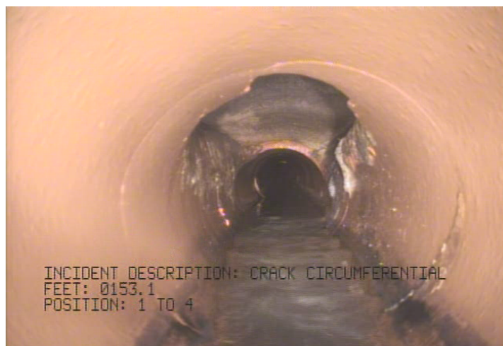
CC - Crack Circumferential @ 153.1 ft.
