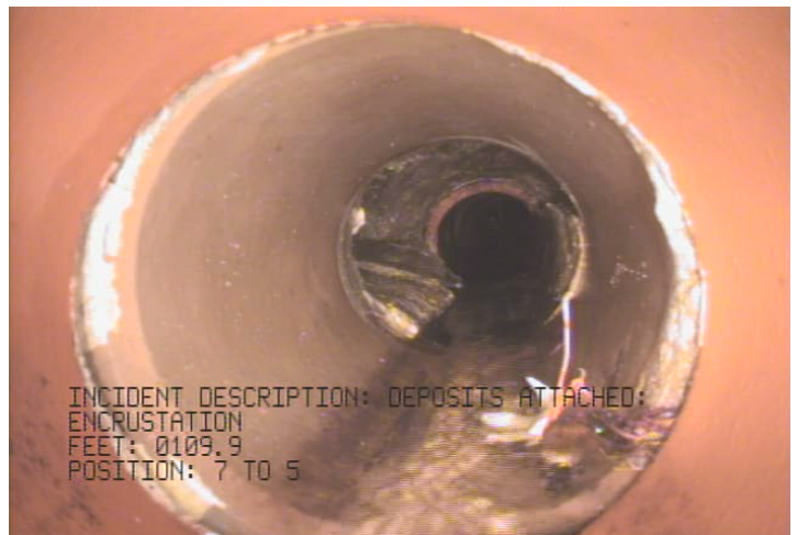
DAE - Deposits Attached: Encrustation @ 109.4 ft.
