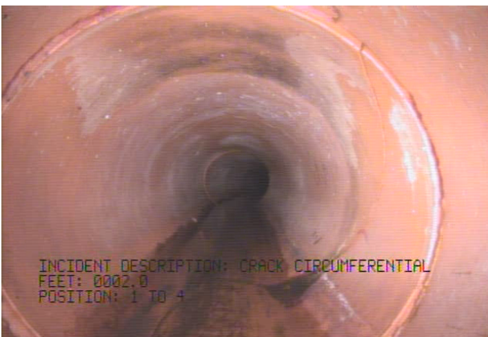
CC - Crack Circumferential @ 2.0 ft.
