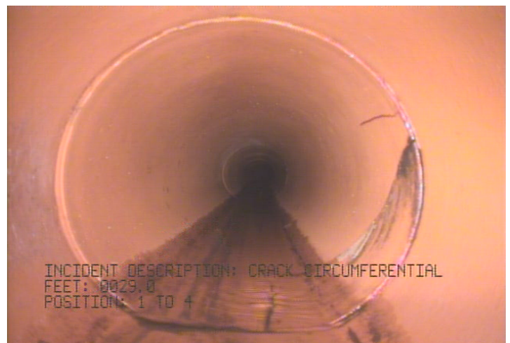
CC - Crack Circumferential @ 29.0 ft.
