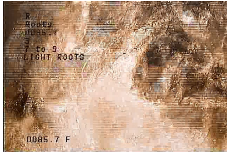
L - Lateral @ 119.4 ft. STUB
