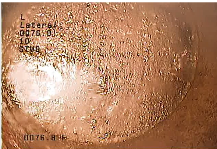
L - Lateral @ 76.8 ft. STUB
