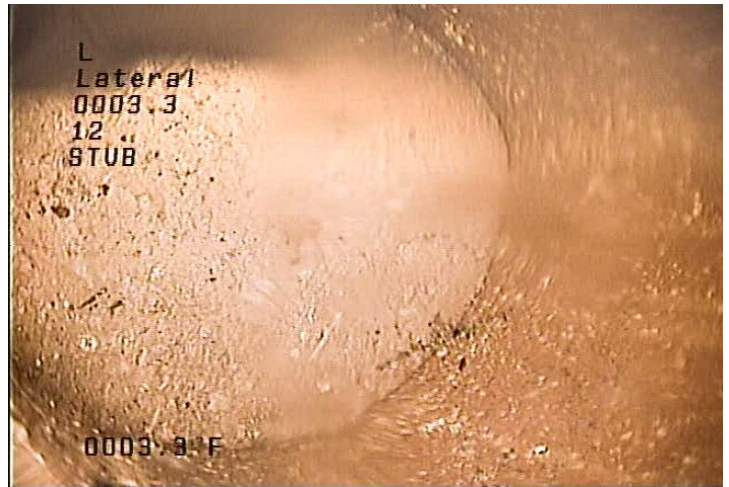
L - Lateral @ 3.3 ft. STUB
