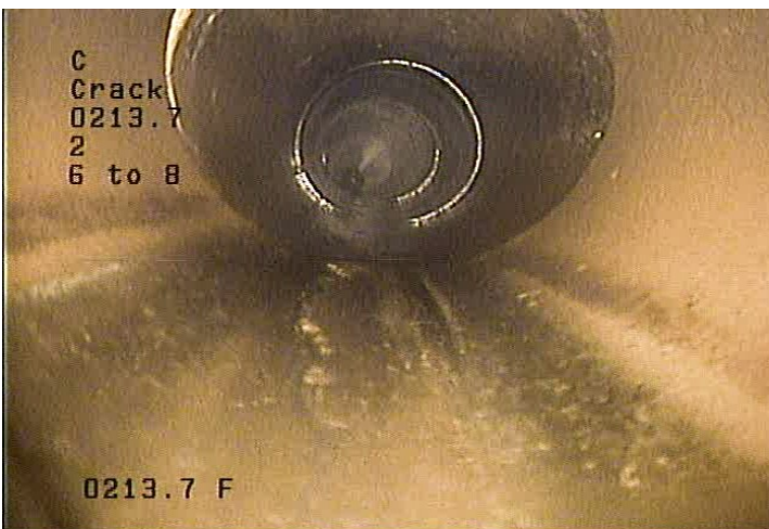
C - Crack @ 213.7 ft.
