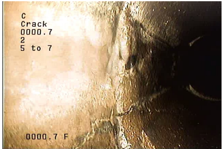
C - Crack @ 0.7 ft.
