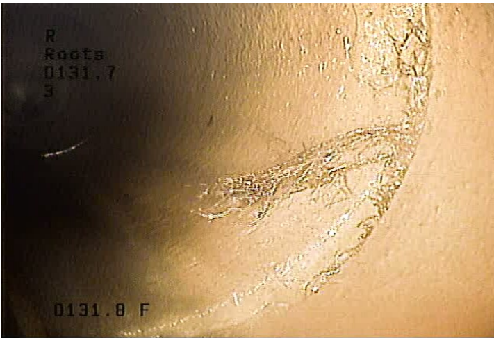
C - Crack @ 138.2 ft.
