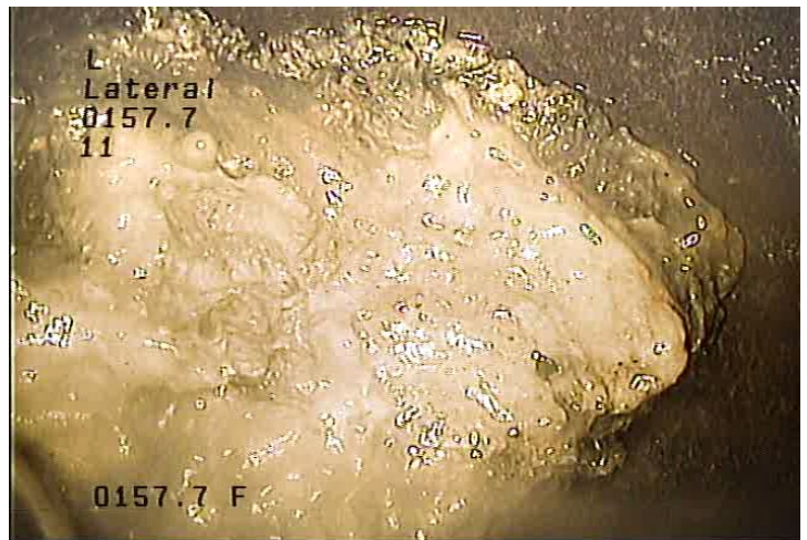
C - Crack @ 196.7 ft.
