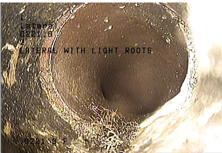
L - Lateral @ 221.8 ft. LATERAL WITH LIGHT ROOTS
